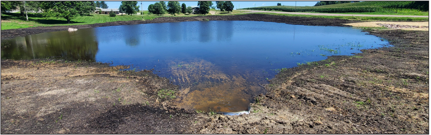
Contractors in summer 2020 excavated more of the wetland to increase flood storage, and installed a culvert connecting it to the upper watershed.
